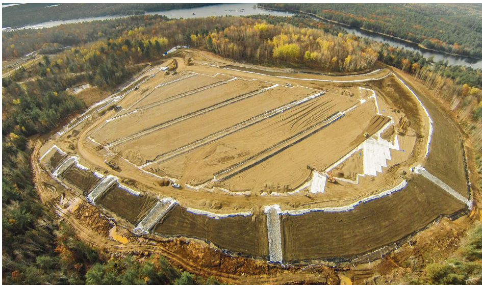
Area B nearing completion. The site has been levelled and geosynthetic clay liner is being backfilled with local silt.
