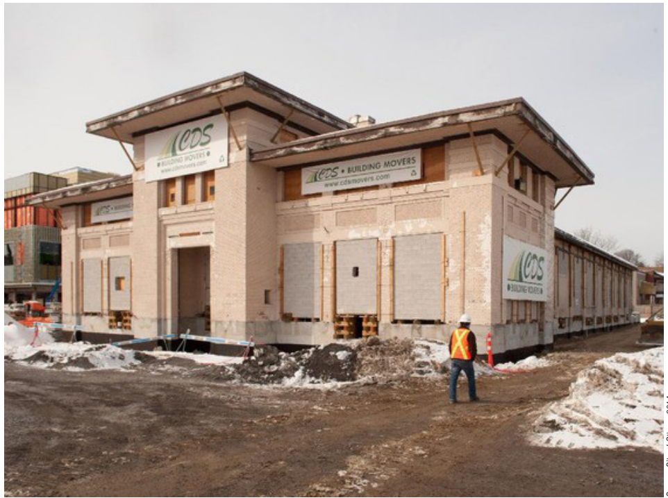
Renovations and relocation of the Horticulture Building at Lansdowne Park, Ottawa, ON.
