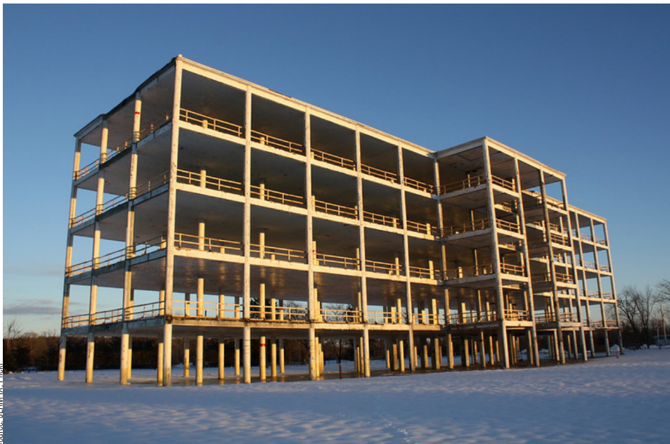
Photo of the Bata Shoe Factory demolition in February 2014, showing exposed building interior and floor slabs 37 .
